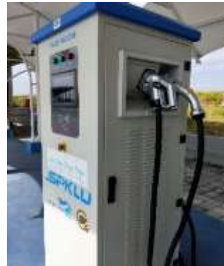
Gambar 6. Fast public charging station di Kota Denpasar [12]
