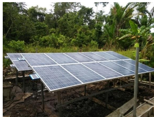
Gambar 1. Pompa Air Tenaga Surya [5]
