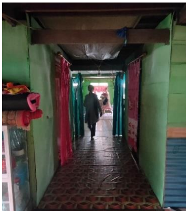
Figure 9. The position of the door is not according to the rules
