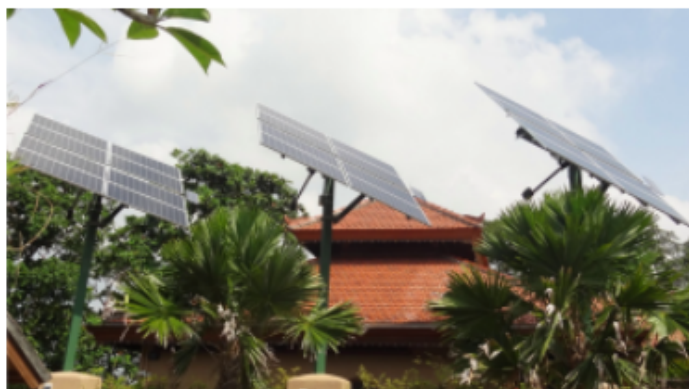
Gambar 4: Sistem PLTS Botha Villas Sanur kapasitas 5,76 kWp [10]
