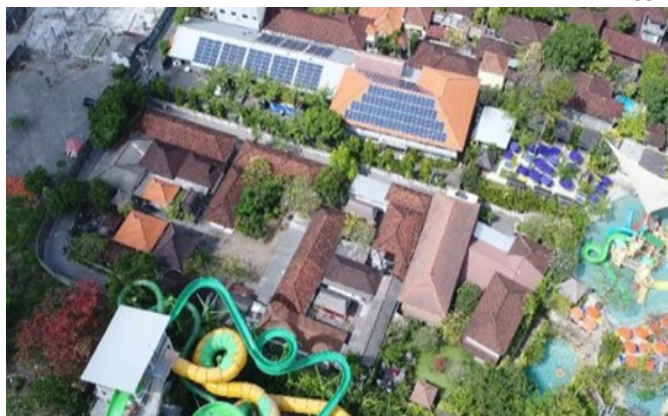
Gambar 12: PLTS on-grid Waterboom Bali kapasitas 156,09 kWp [13]
