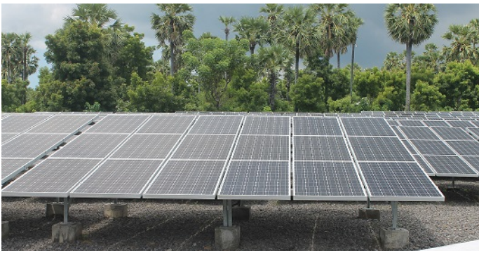
Gambar 5: Sistem PLTS On-grid Karangasem kapasitas 1 MWp
