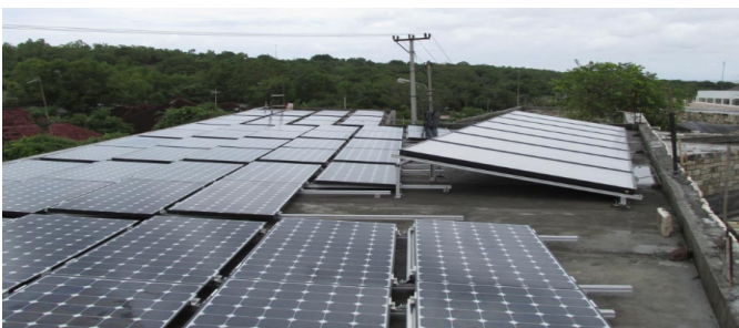
Gambar 7: Sistem PLTS Off-grid Suarga Resort kapasitas 70 kWp [11]
