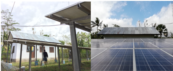
Gambar 1. PLTS off-grid 15 kWp Datasah
