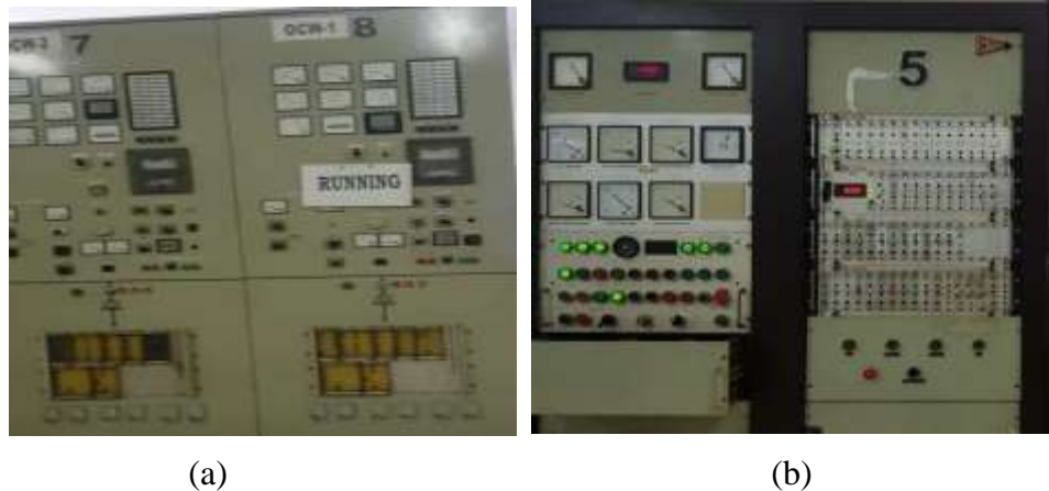
Gambar 1. (a) Generator Control Panel , dan (b) Engine Control Panel
