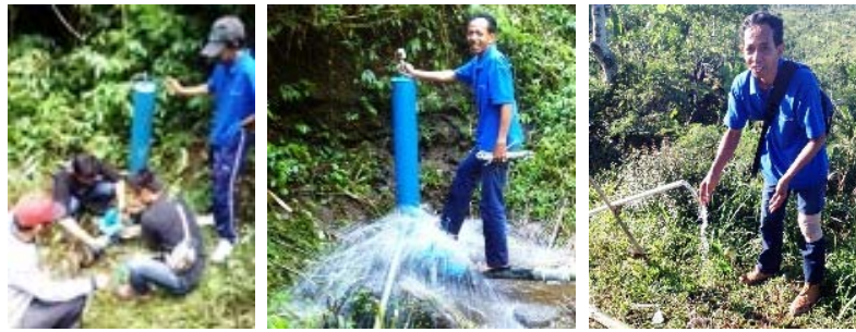
Gambar 4.2. Uji coba operasional pompa hydram
