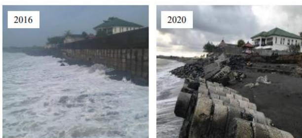
Figure 1 The existing revetment on the Tegal Besar beach in 2016 and year 2020
