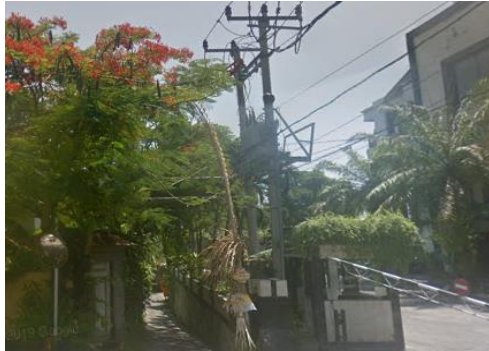
Gambar 1 Gardu Listrik Umalas Hotel dan Residence Sumber: Anonim (2019)
