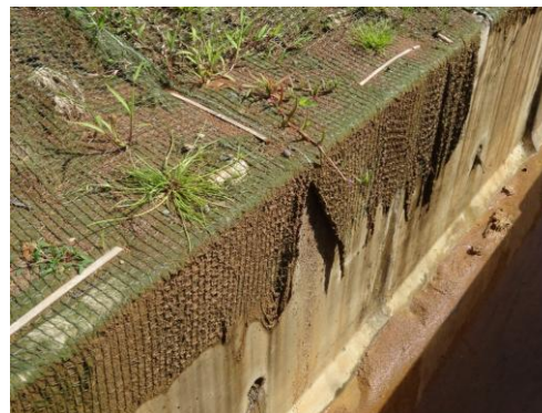
Figure 13. Condition in the drainage channel under another similar sheet covered plot after 3 months
