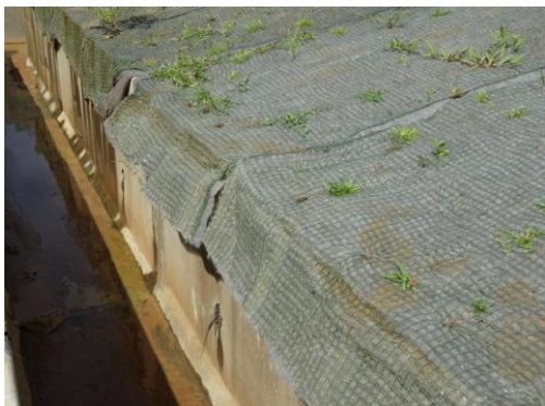
Figure 12. Condition in the drainage channel under the sheet covered plot after 3 months
