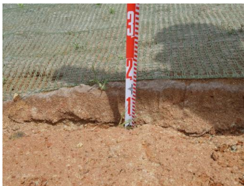
Figure 18. Level difference in the border line between the sheet covered plot and the neighbor bare plot after 2 months
