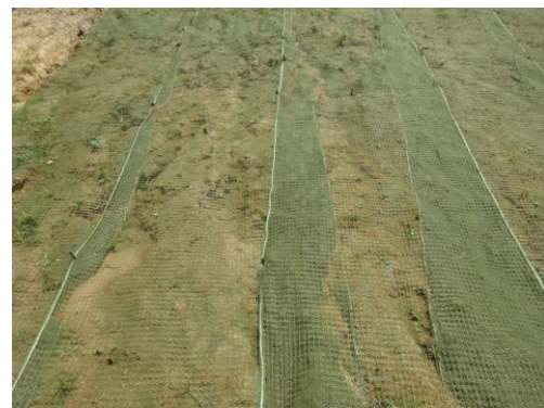
Figure 19. Appearance of soil erosion beneath another similar sheet after 2 months
