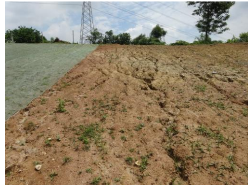
Figure 17. Appearance of the gully erosion occurred in the bare part of the neighbor of the sheet covered plot
