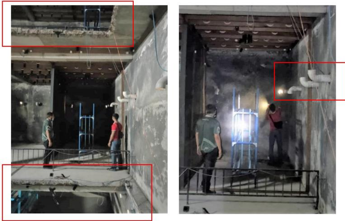
Figure 4. Large Opening in Certain Floor (passage of swiftlets) (left) and Air Ducts (right)
