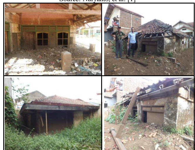
Fig. 3 Houses destroyed by floods in Cieunteung village Source: Nuryanto, et al. [1]
