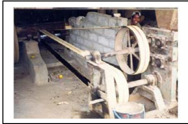
Figure 8 Pulley belts without appropriate safety protective
